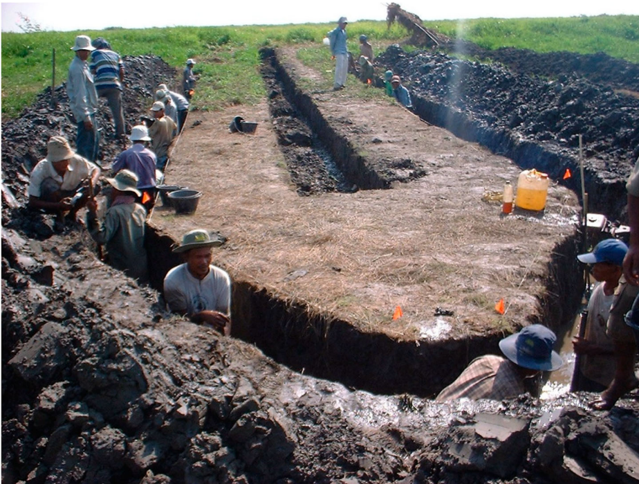
Figure 1. Excavation across Paris Canal 4, linking the historic centres of Angkor Borei (Cambodia) and Oc Eo (Vietnam), on the upper Mekong River delta in southern Cambodia (March 2004). The encircling drainage trench, from which water was continuously pumped, created a local depression in the groundwater table that preserved the integrity of the research trench (centre), allowing a nearly 2 m deep excavation to the base of the canal infill. Photo: Dan Penny.
